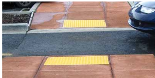
Illegal placement, not enough coverage
