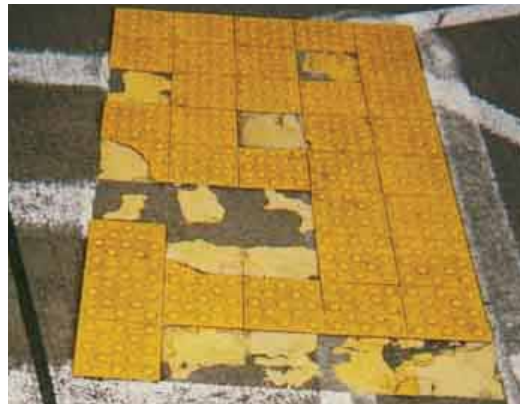
Glue Down Delamination
