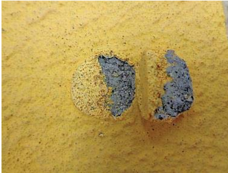
Photo No. 11 Bond Strength Failure Detail
